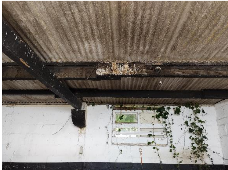
Figure 21: B3 Corrugated cement roof and evidence of nesting birds
