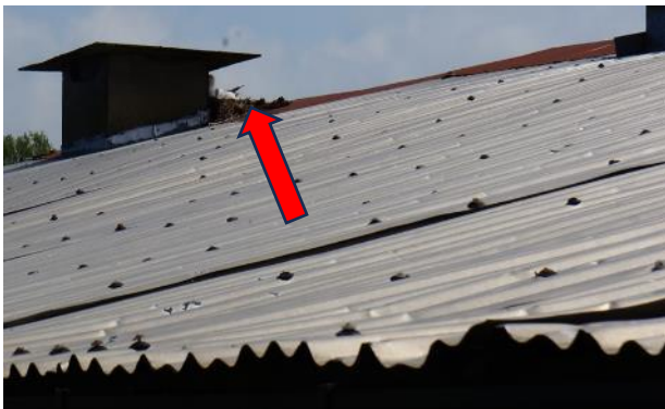
Figure 15: Gull nesting on the roof of B9.
