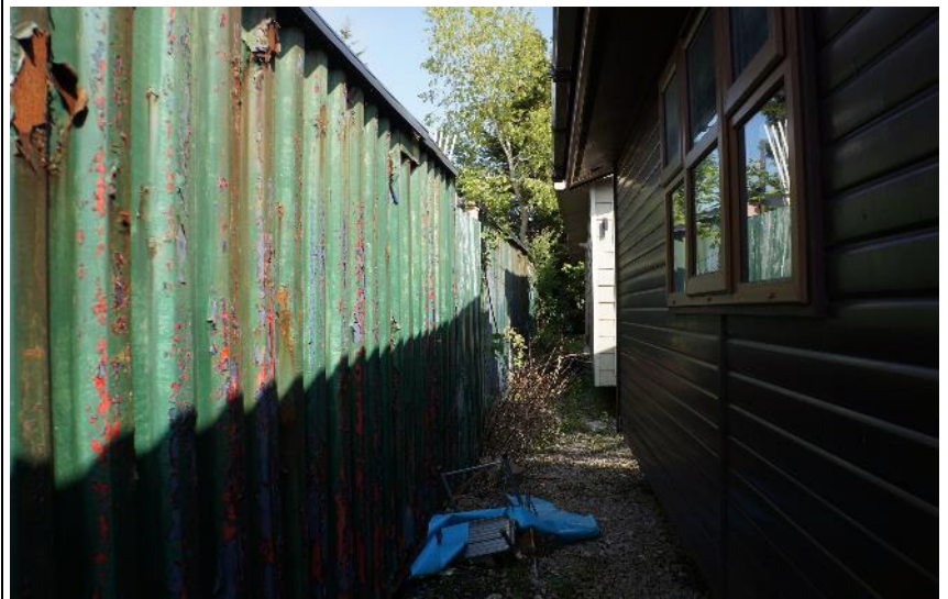
Figure 29: South elevation of B17, with static caravans to the right of view.
