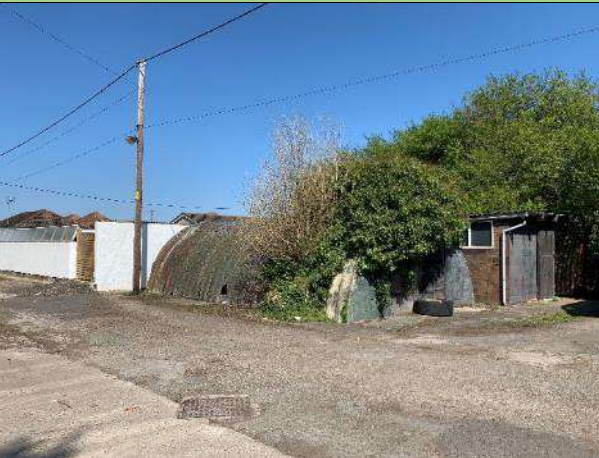
P23: A manhole and a unit with suspected asbestos sheet roofing in the north-east of the site. Photo facing north-east.
