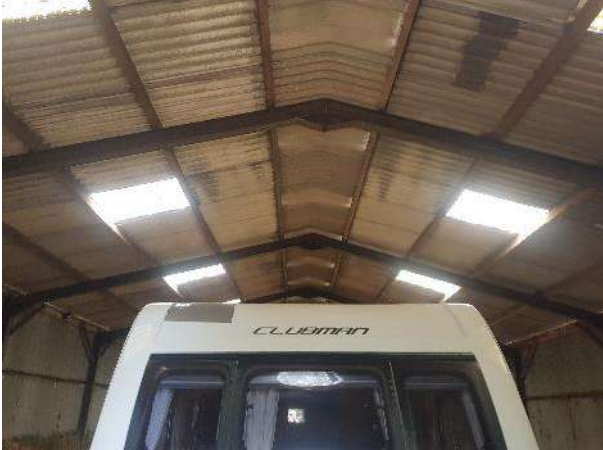
P15: View inside the aforementioned unit showing the suspected asbestos roofing.
