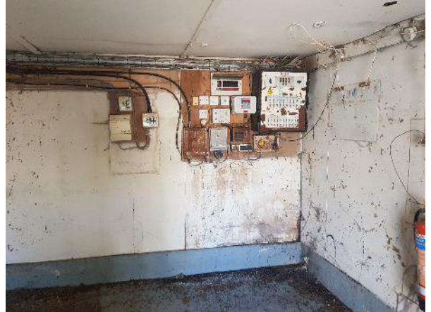
P10: Electrical unit within the entrance to the southernmost poultry house.
