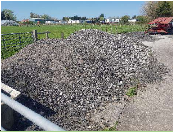
P7: Pile of coarse aggregate near the south-western corner of the southern section of the site.
