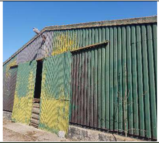
P14: A unit with suspected asbestos sheet roofing located in the east of the site.
